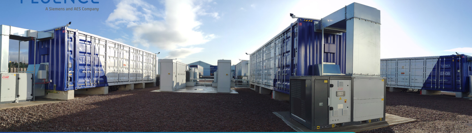
Fluence Advancion Deployment
