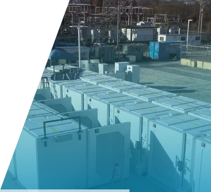
The Fluence Systems Test Lab in Pennsylvania, USA serves as the primary location for system-level testing of various configurations of our energy storage products.
